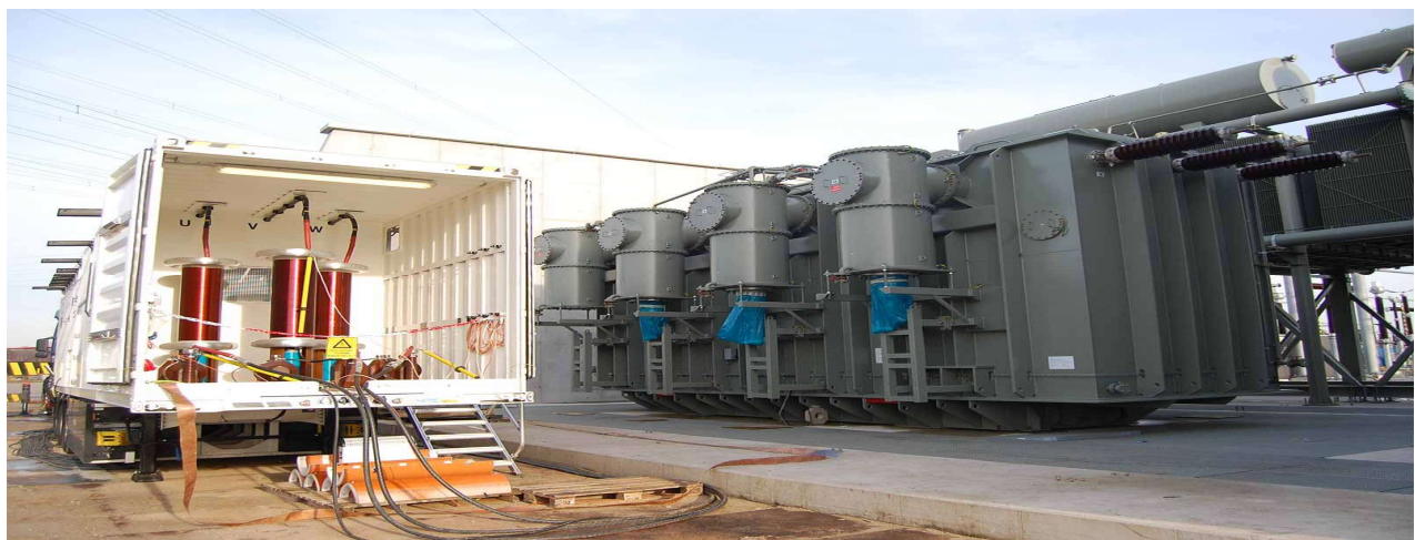
HV Test for Power transformer
